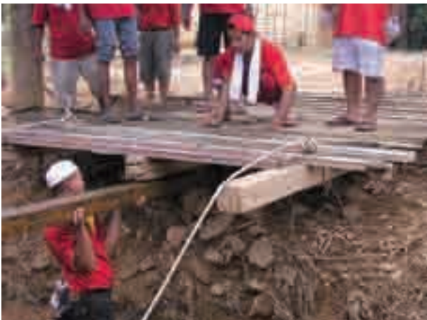
The AmBank Group staff members helping to repair a bridge connecting a few houses to the main road in Kampung Batu 25, Johor.
